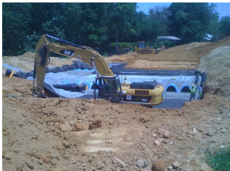
Figure 1: Stormwater Management System
